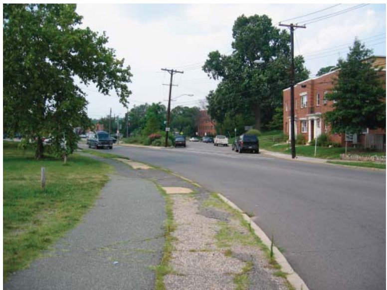
Poorly maintained sidewalk – 10 th Street south of Michigan Avenue
