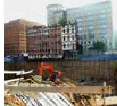
Construction activity for development and public infrastructure requires strong leadership and commitment of resources.
